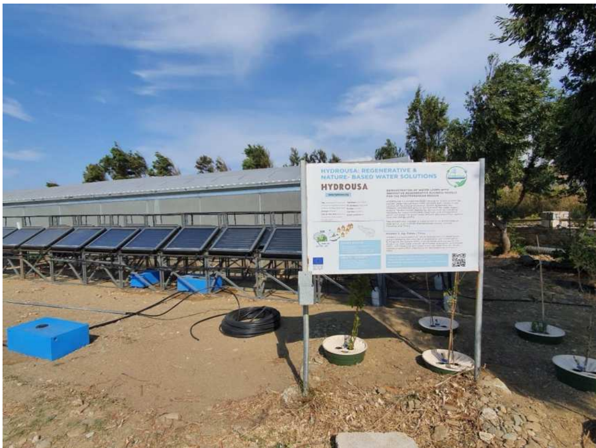
Figure 2.7 Desalination system coupled with the tropical greenhouse
